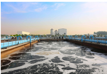
Industrial Water Treatment
